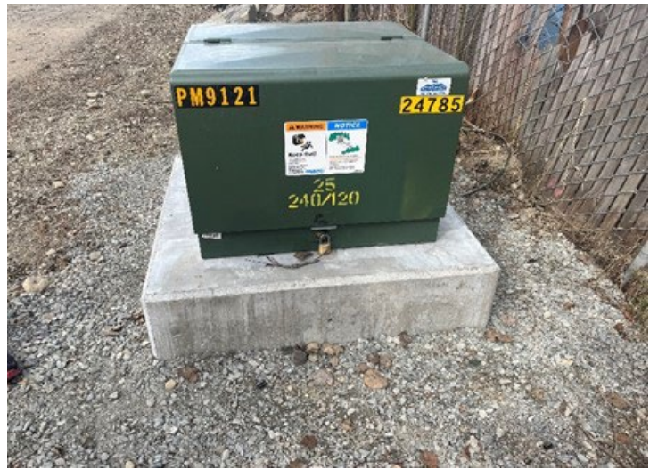
Photo 2. Pad-Mounted Transformer Along N Side of Property
